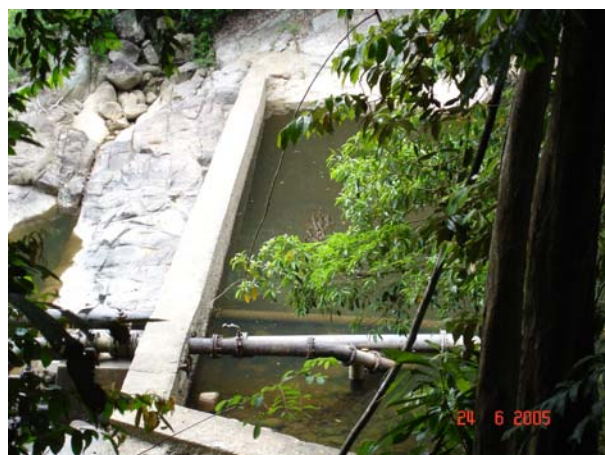
Figure 1. Water treatment plant at Hin Lad
