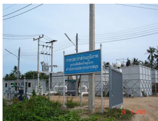
Figure 9. Mobile water treatment plant at Chaweng
