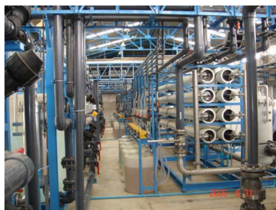
Figure 8. RO System water treatment plant at Bo Phut
