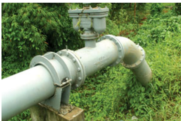
Figure 10. Existing water supply distribution pipeline
